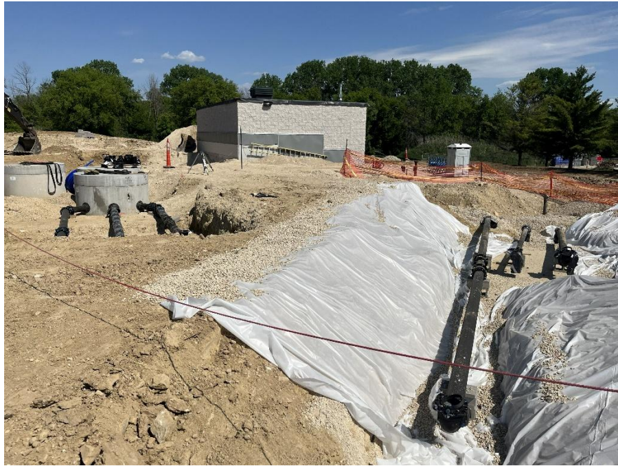
STR 600 underground piping.
