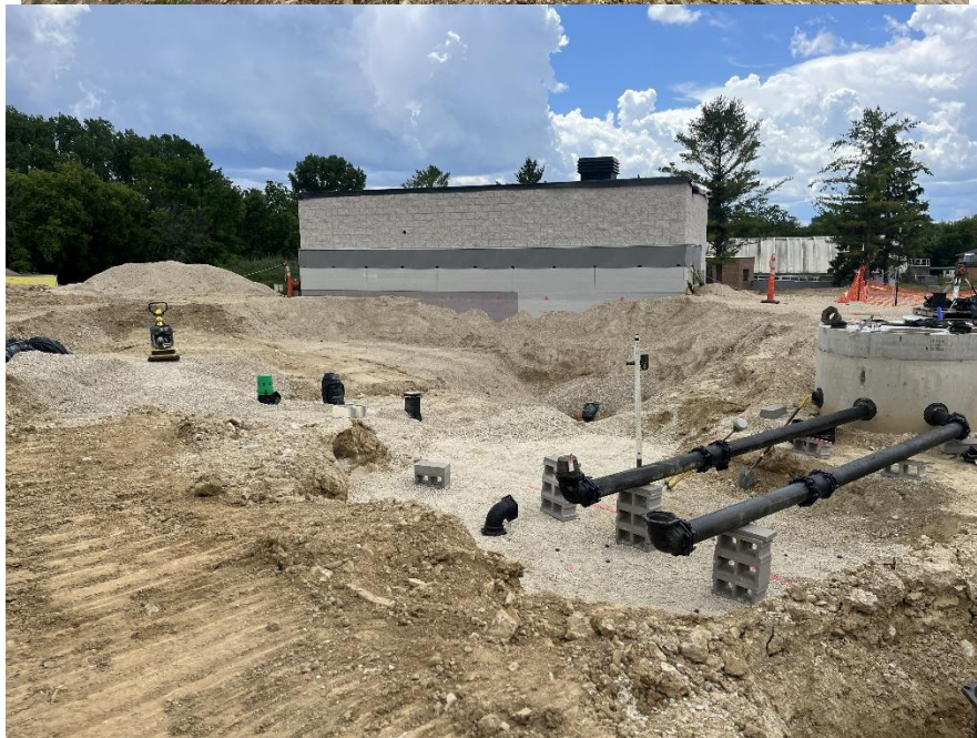
STR 700 underground piping.
