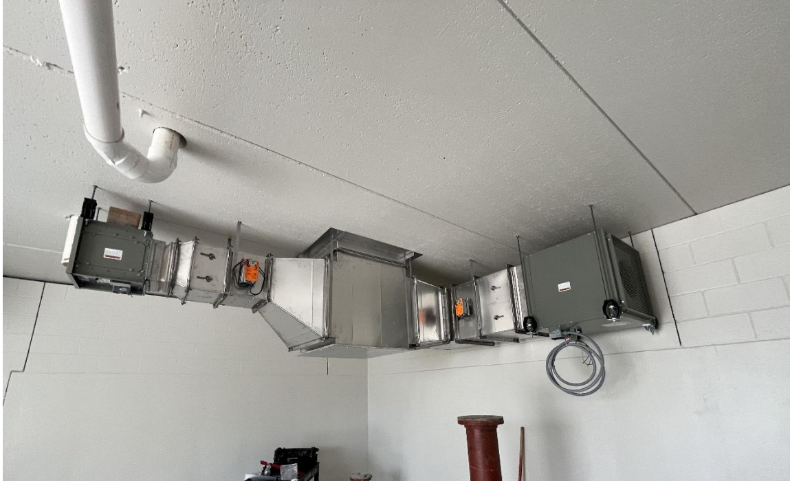
STR 650 HVAC and louvre installed.
