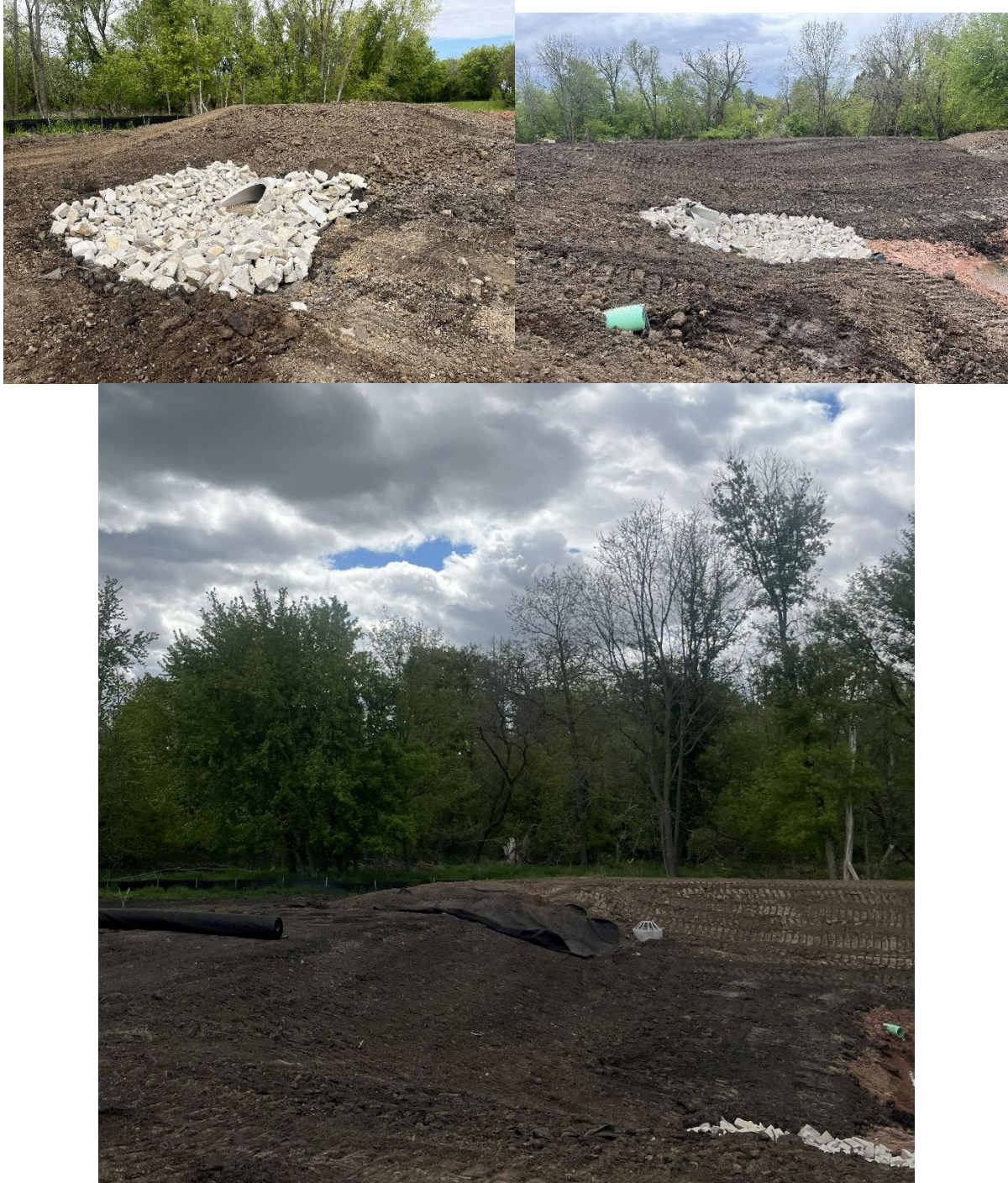
Rip Rap installed in West Wet Pond near STR 800, overflow spillway beginning to be lined.
