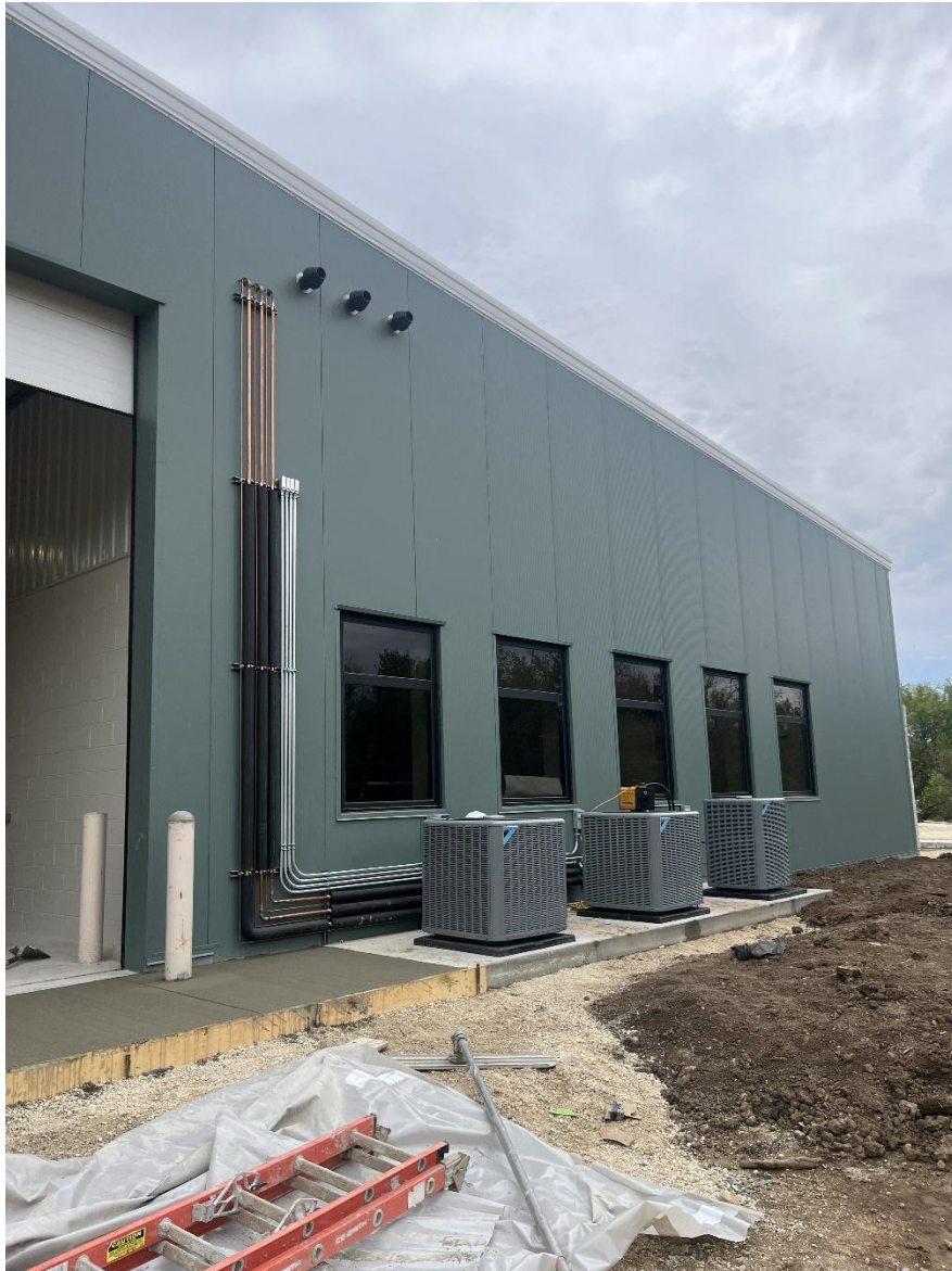
STR 800 HVAC/Condensing units installed.
