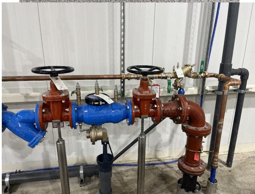
STR 800 DI/RO System Installed and Tagged. Non Potable Water system installed and tagged.
