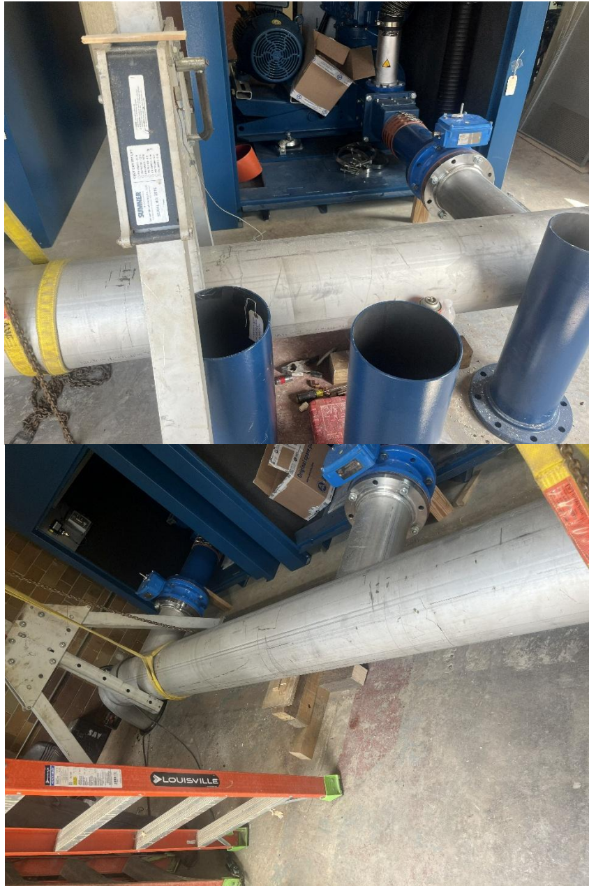
Blower piping in STR 100, connected to blowers and through floor.
