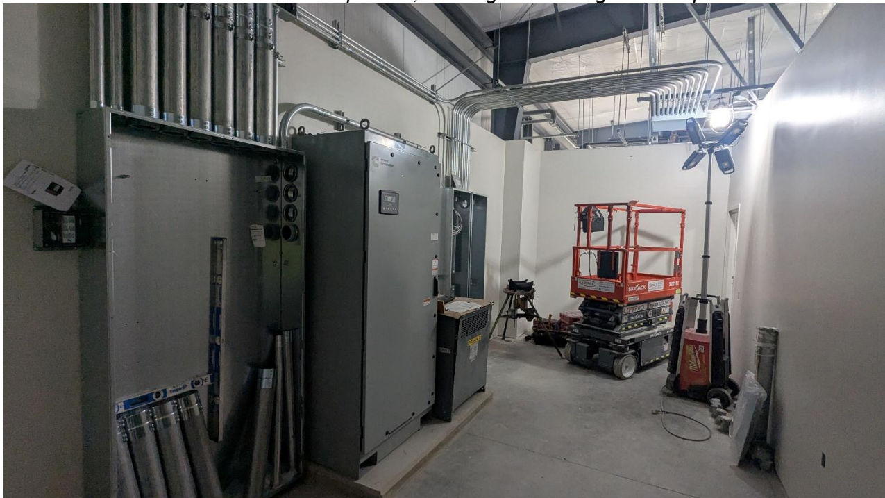
STR 800 electrical equipment installed, walls painted
