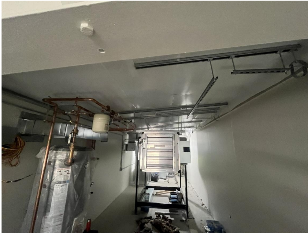
HVAC installed in STR 800 Mezzanine. Lighting to be installed.
